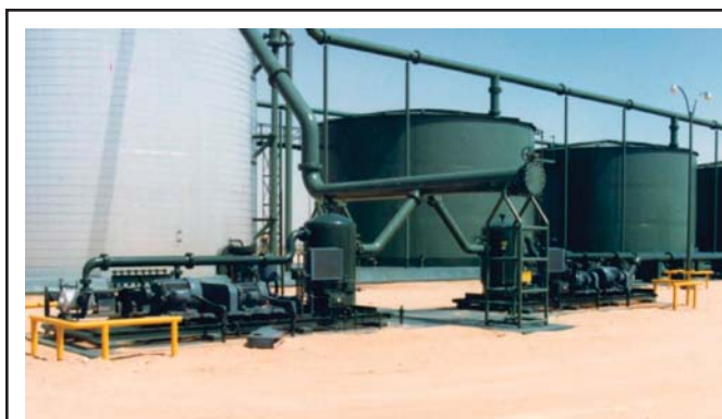
The combination of advancements in vapor recovery technology and strong natural gas prices are making VRU applications very economic, typically providing payback of capital equipment costs in less than six months.
