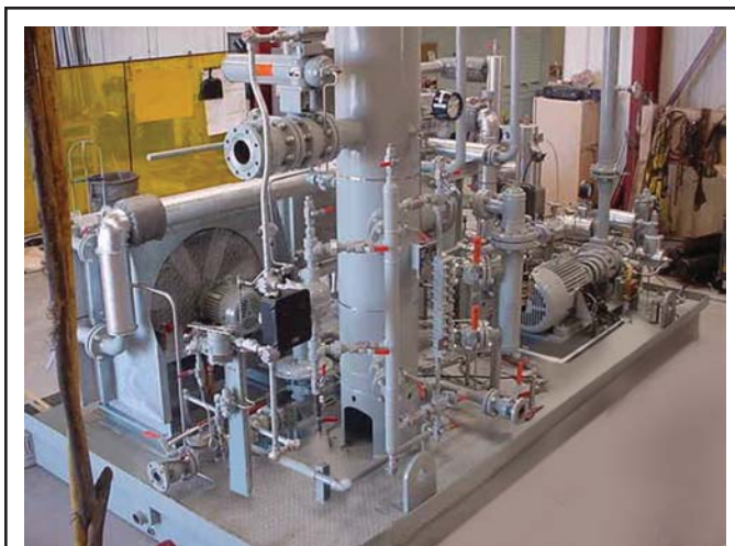
The compressor is a critical element in VRU system design. Rotary screw or rotary vane compressors are best suited to vapor recovery applications because of their ability to effectively handle wet gas. Shown here is a VRU installed on an offshore platform.
