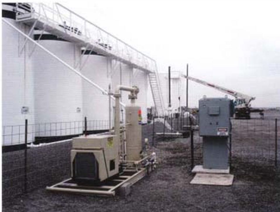
A vapor recovery system on location uses a new Emerson Scroll compressor and a fully-automated programmable logic controller (PLC) system, which allows the system to effectively capture a wet, low-pressure gas stream.
