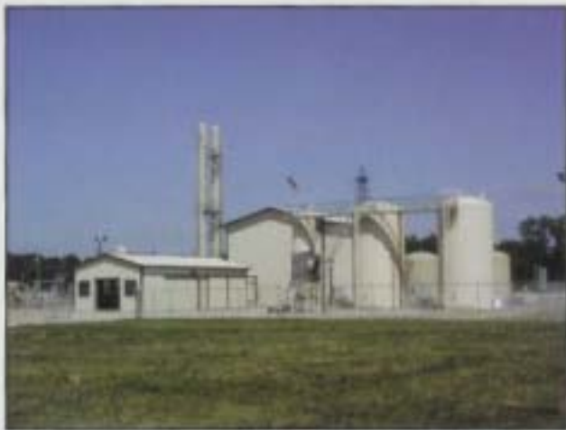
■ Salem Plant's bio-desulfurization plant uses microbes to digest and convert H 2 S into elemental sulfur.
