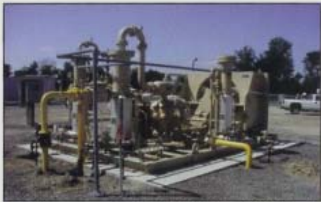
■ The plant compressor is a Gemini A-352, 250 hp (186 kW) electric drive/two-stage recip.
