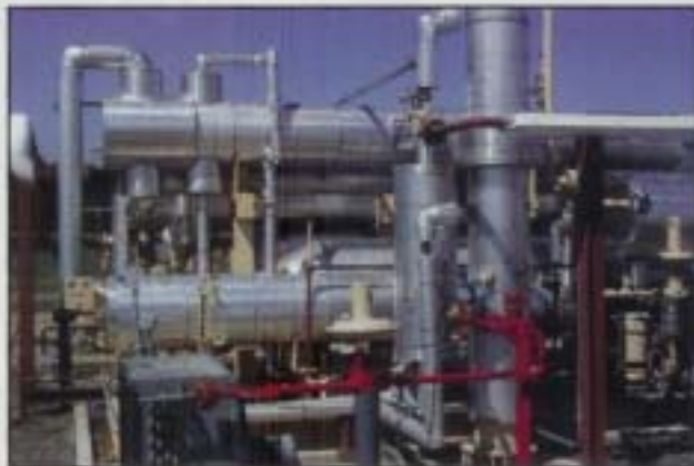
■ The mechanical refrigeration unit chills gas to -20°F (-28°C).
