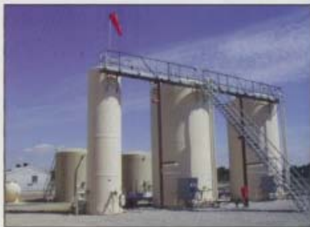
■ The Salem Plant pump tank and two bioreactors.
