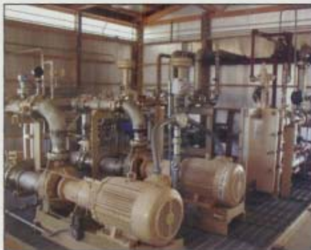
■ The NAOH solution circulation pumps for bio-plant.
