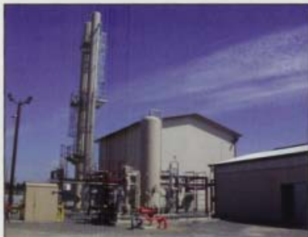
■ The contactor towers for bio-plant are 65 ft. (20 m) tall.
